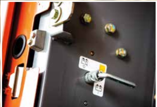
The disconnect switch has improved safety during maintenance.
